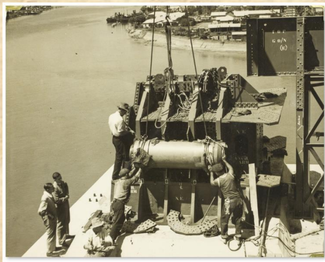
Placing the main pin, Story Bridge Placing the main pin, Story Bridge, c1939; Joe Lang at left, standing, wearing hat. (John Oxley Library collection)
